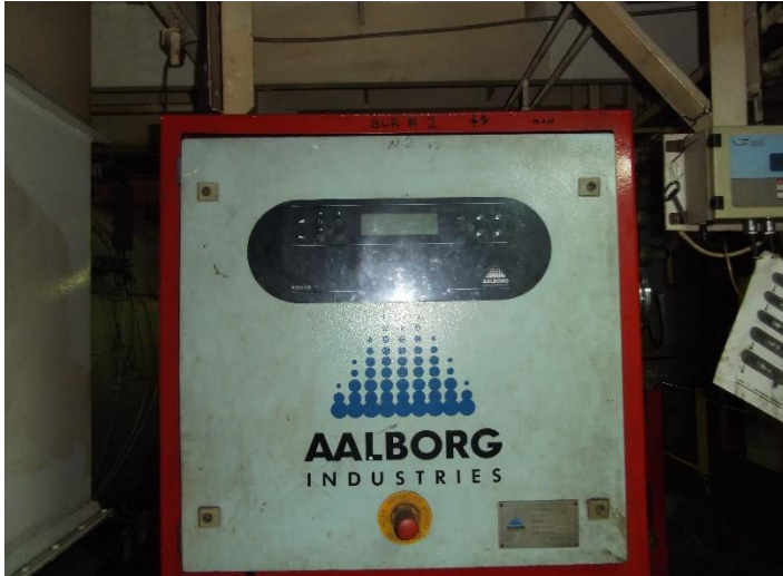
Boiler Local panel
