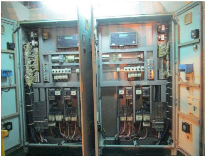
Boiler power panel, 2 Unisab inside
